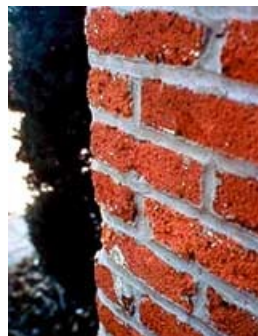
Abrasive cleaning methods like sandblasting can cause significant damage to historic materials
